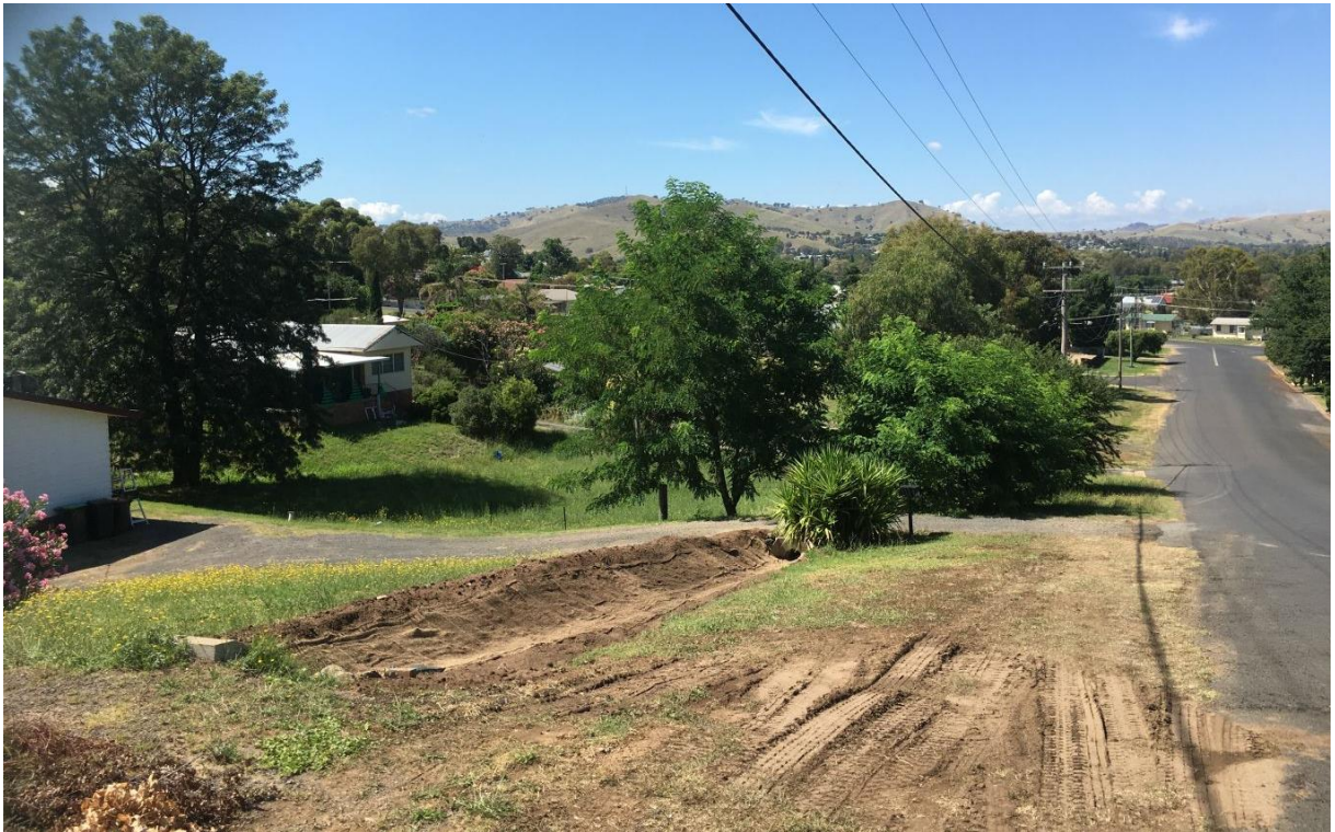
Figure 6 – Inadequate roadside drainage. Tor St Gundagai (G1)
