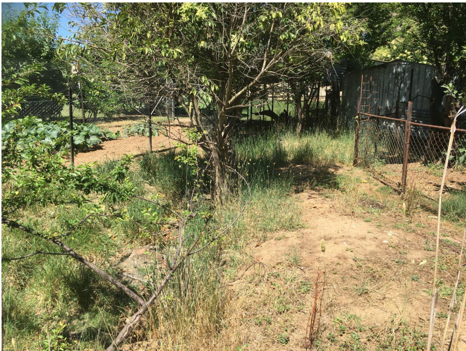
Figure 7 – Stormwater drainage through private property between Tor St and O'Hagan St, Gundagai (G5)
