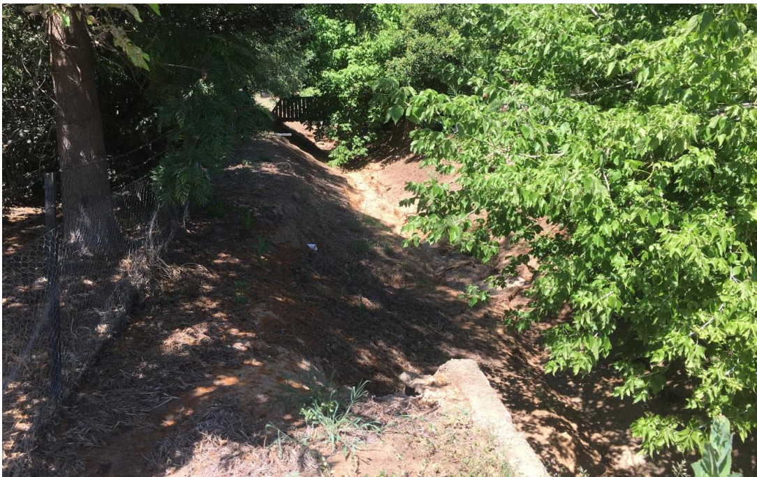
Figure 9 – Open drains through private property. Middle St South Gundagai (G9)
